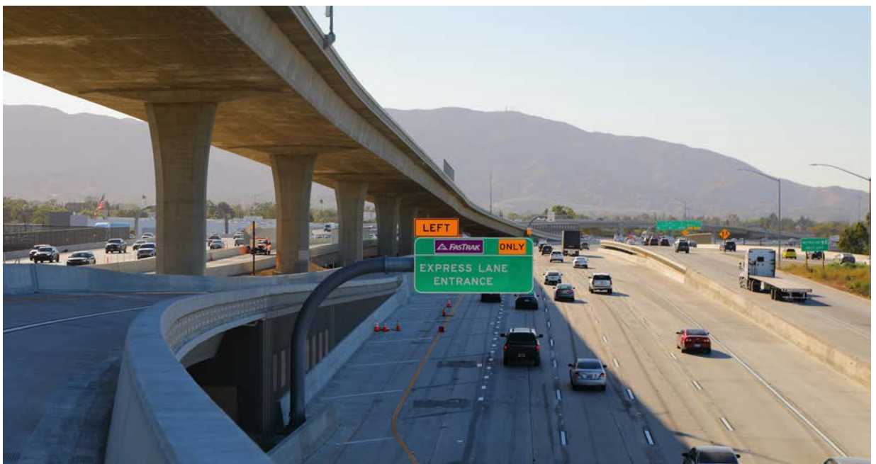
New Southbound 15 to westbound 91 Express Lane Connector overlooking 91 Express Lanes in Corona
