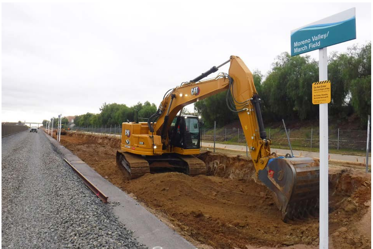
In fall 2022, crews began upgrades to the Moreno Valley/March Field Station in Riverside.
