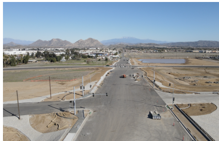
Intersection lights installed at northbound I-215 on- and off-ramp and Placentia Ave.
