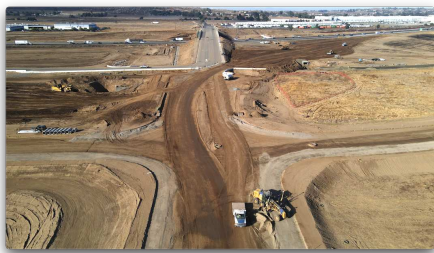
Future intersection of Placentia Ave. and the new E. Frontage Rd. alignment.
