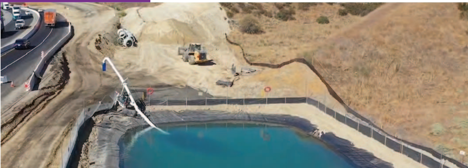
Crews have built two temporary water reservoirs to provide a local water supply for dust control.
