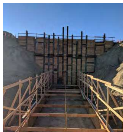
Two wildlife crossings are being built to provide safe passage for animals under the roadway.
