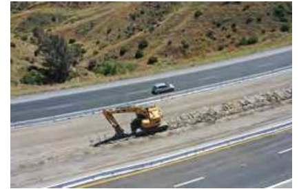
Crews are excavating the center barriers to increase space for additional lanes.
